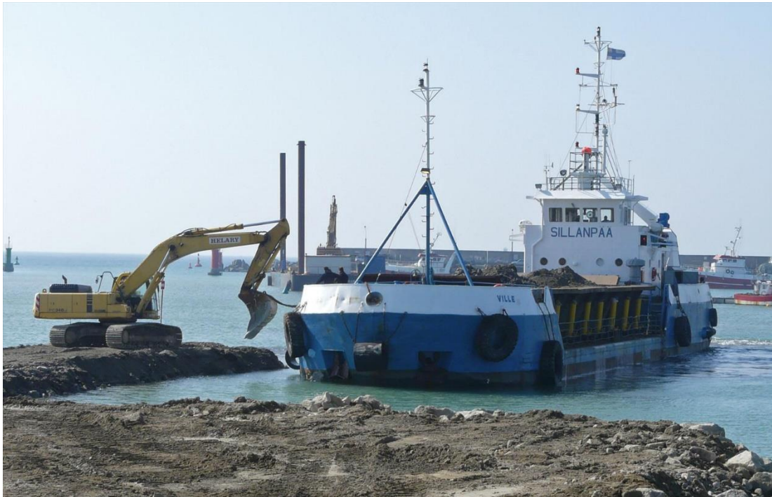
Tipping the rocks directly on site – below and above the water, where the rocks must be used.
